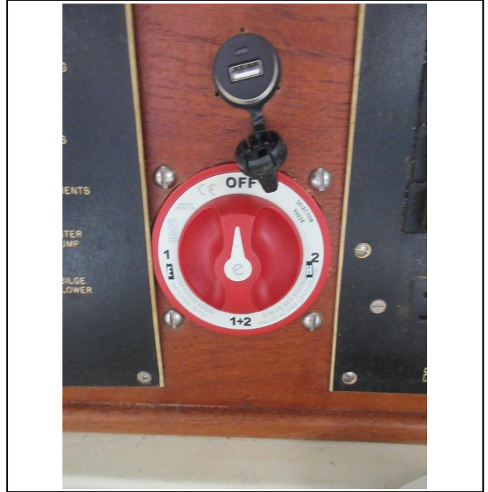
Main Battery Switch
